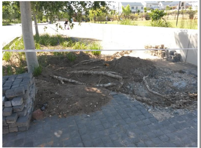
Photo 14: Tree roots from the road-side poplars are causing lifting of pavement surfaces.
